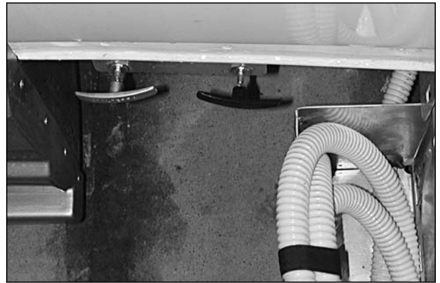
Picture B-P27: Black water, grey water valves and sewage hose locations.
